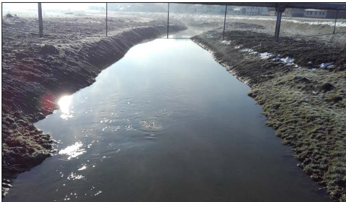
Figure 1b: Human impact on the Hârtibaciu River studied sector on banks and riverbed.
